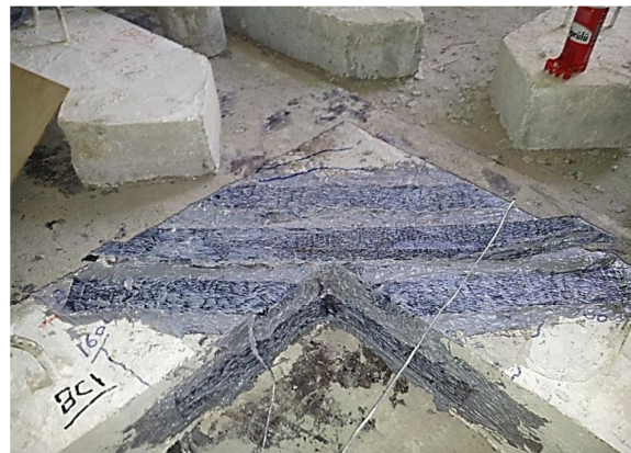
Fig.(4) Crack pattern of the specimen preloaded until 80% ultimate load and strengthened with strip of CFRP (BC1)
