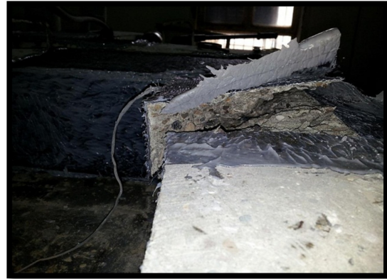
Fig.(8) Delamination of concrete cover for specimen preloaded until first crack load and strengthened with full-CFRP (BC16)
